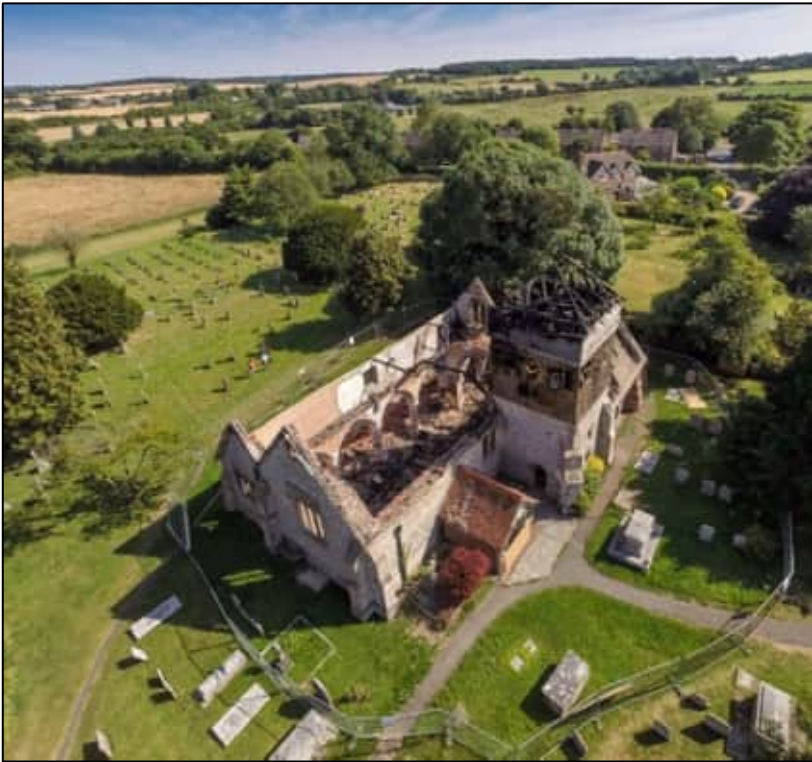
Aerial view of the church, left gutted following the fire
